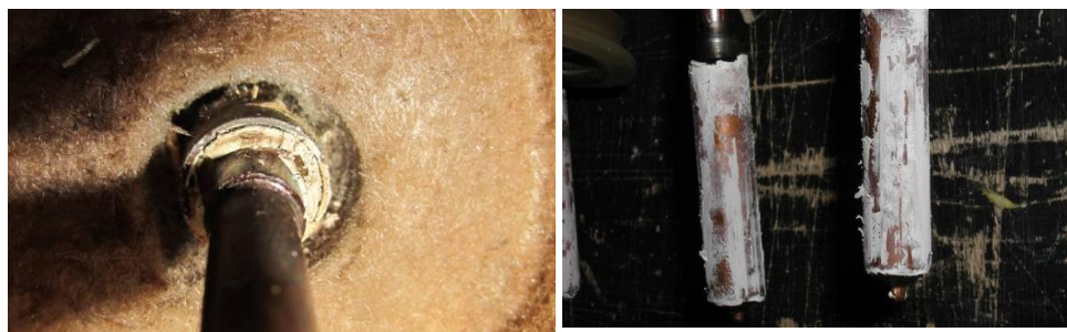
Picture 4: 137-10/KP Koll 2 non removable connection of heat pipe to manifold after final performance test
