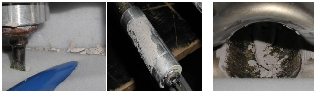
1) traces of heat transfer paste in manifold casing before starting interim performance test 2) Condenser 3) manifold after final performance test, before renewing the heat transfer paste
