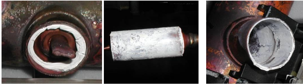
Picture 6-8: 68-11/KP Koll 1 Condenser and manifold after final performance test before renewing the heat transfer paste
